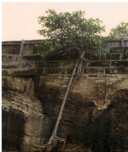
Tree growing out of a retaining wall
